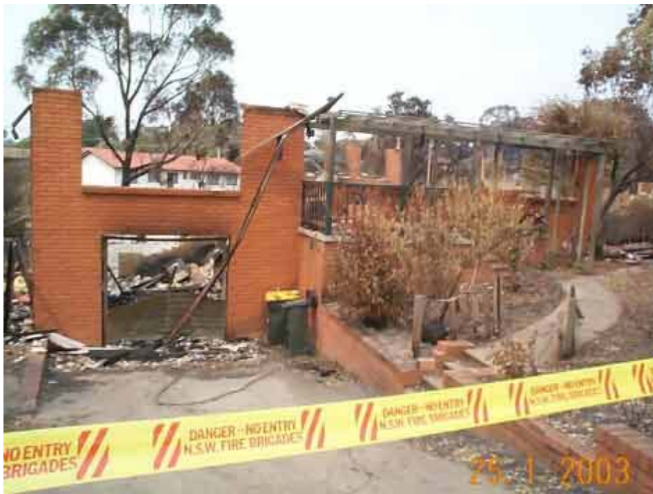
Houses in Duffy did not stand a chance once the windows were blown in.
