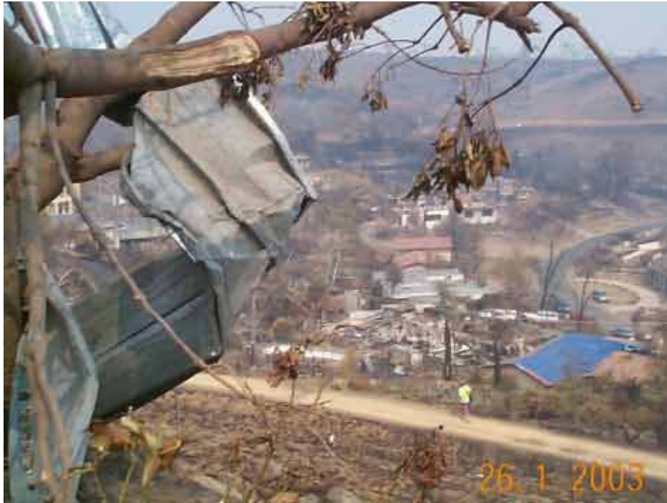
Roofing materials were found hundreds of metres from original dwellings.
