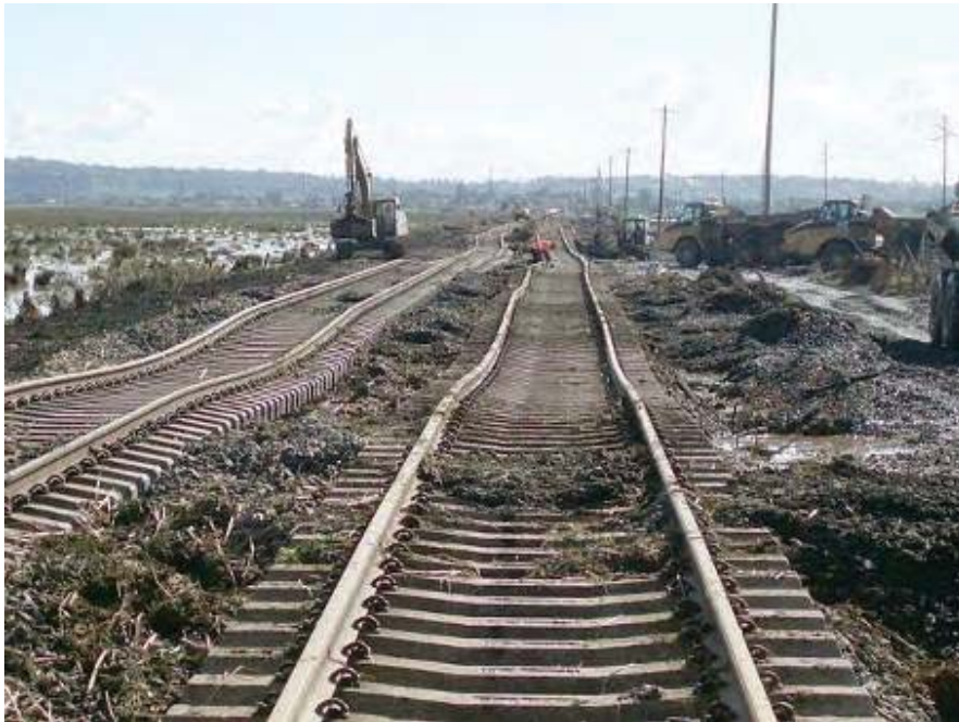
Figure 14 Damage to the rail lines as a result of the heavy rainfall and subsequent erosion (source: Australian Rail Track Corporation)
