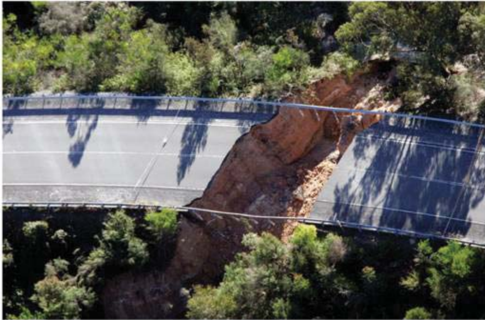
Figure 13 Collapse of Pacific Highway, Somersby Central Coast (source: ABC TV)
