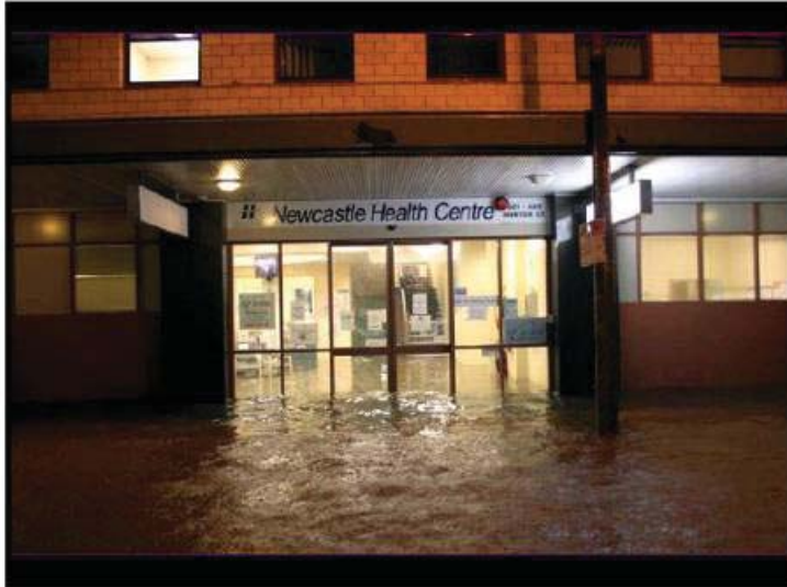
Figure 15 Damage sustained to health facilities during the flash flooding in Newcastle (photo courtesy of NSW Government)
