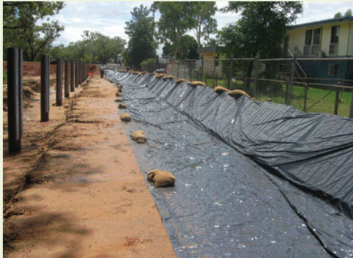
Figure 5: A Constructed Flood Barrier in Charleville, 2008
