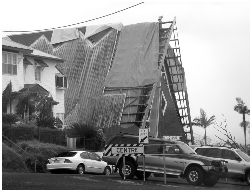
Figure 2:9 'A'-frame roof damage caused by Tropical Cyclone Larry – March 2006
