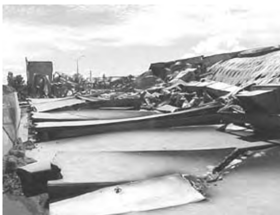
Figure 14:21 An example of a 90 degree angle wall collapse
