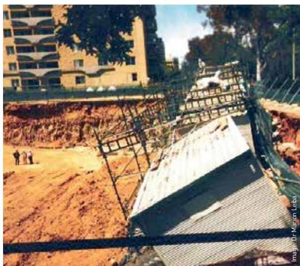
A landslide at a building site in Canberra causes two prefabricated site buildings to come off their foundations.
