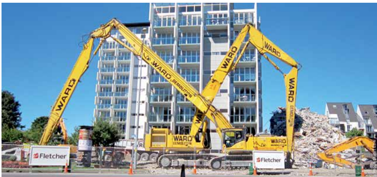
A unit block being 'deconstructed' after the earthquake albeit it remained standing during the event.
