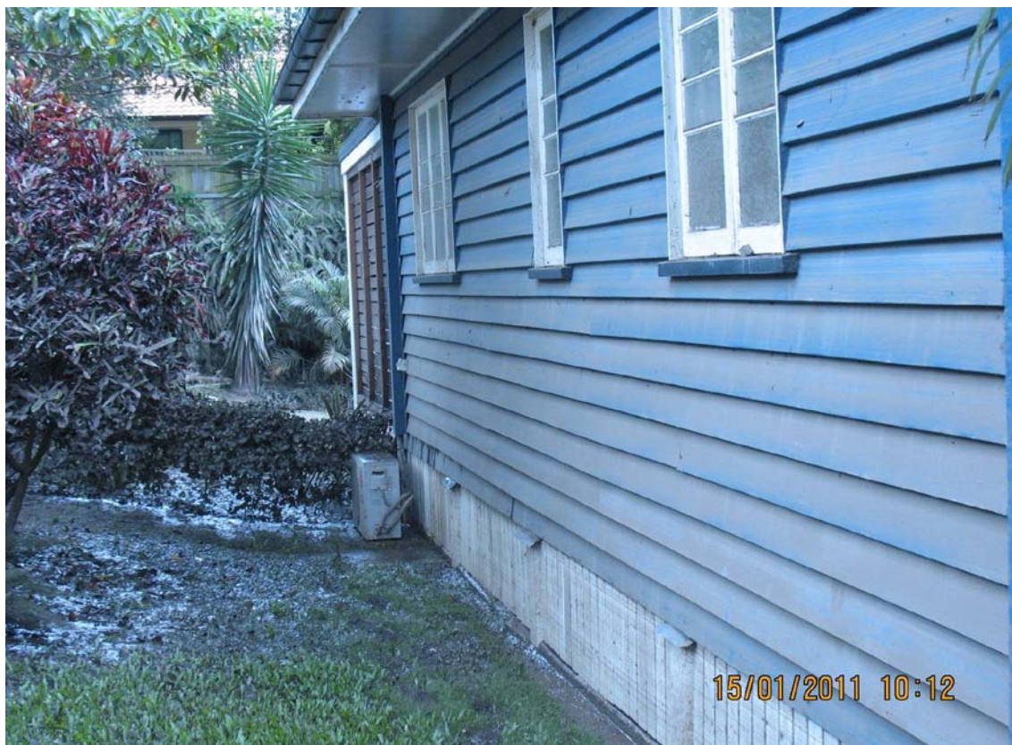
Flood damage in Graceville back yard, neighbouring Graceville Park complex visible over fence (photo courtesy Rob Clements)
