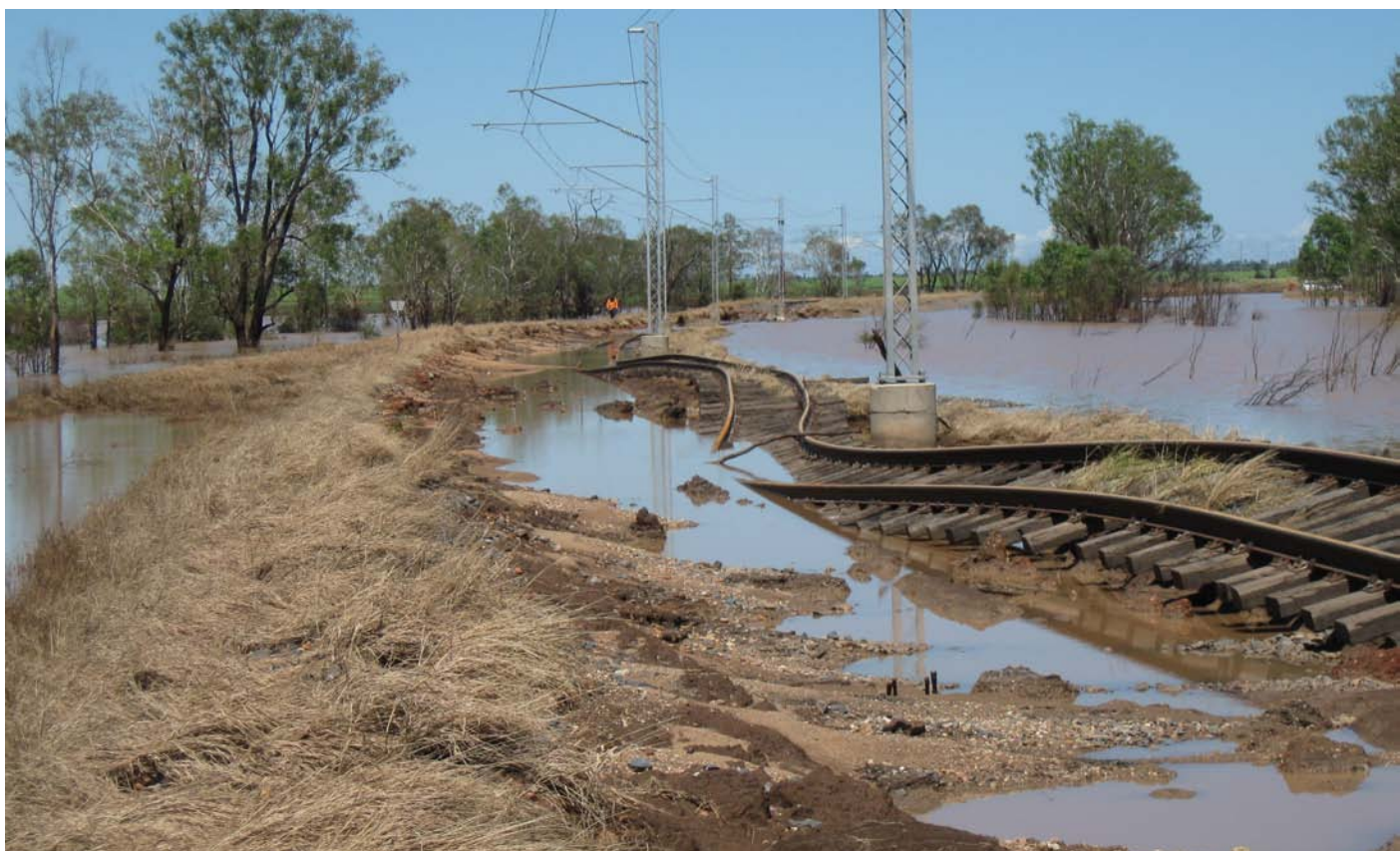
Comet River overflow (photo courtesy QR National)
