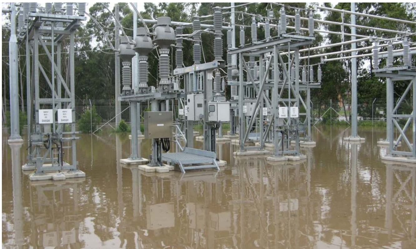
Flooding at Ergon Energy's Bundaberg Central Substation (photo courtesy Ergon Energy)
