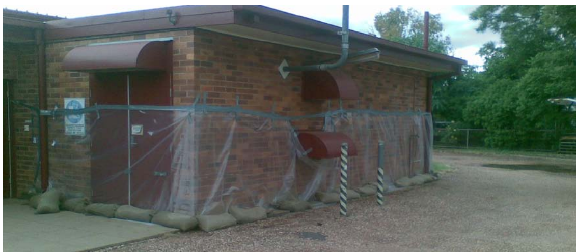
Telstra's St George exchange wrapped in plastic and sandbagged to protect it from floodwaters during the 2010/2011 floods Source: Exhibit 215, Supplementary submission of Telstra, 8 April 2011, Annexure 1 [p9].
