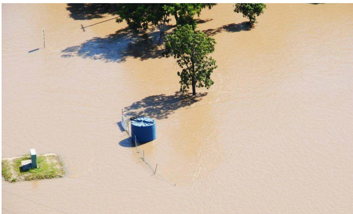
Telstra's CMUX unit at Rockhampton built on an elevated platform, so it was above floodwaters during the 2010/2011 floods Source: Exhibit 215, Supplementary submission of Telstra, 8 April 2011, Annexure 1 [p12].
