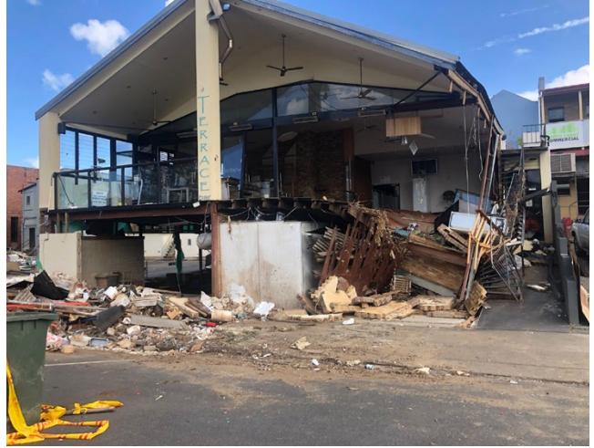
Flood waters swept through the Terrace Bar in Richmond, causing extensive damage.
