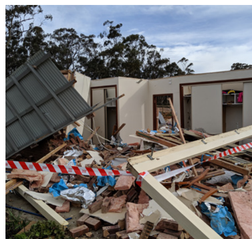
Damage caused by the tornado in Axe Creek, Victoria (12 km southeast Bendigo), 29 June 2019.
