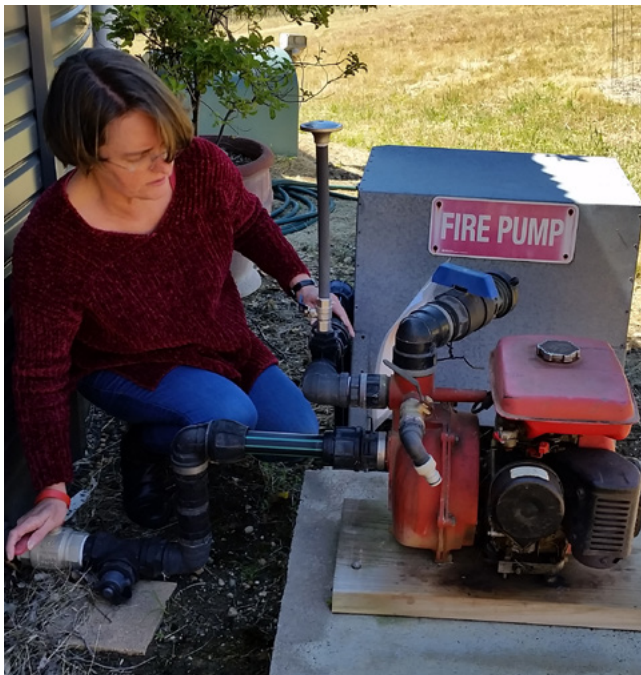
Dr Danielle Clode practising starting her fire pump at her property. Image: supplied by Dr Danielle Clode
